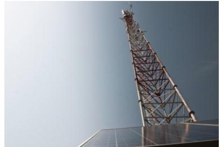
Figure 243: PV-powered telecoms tower in India 4
