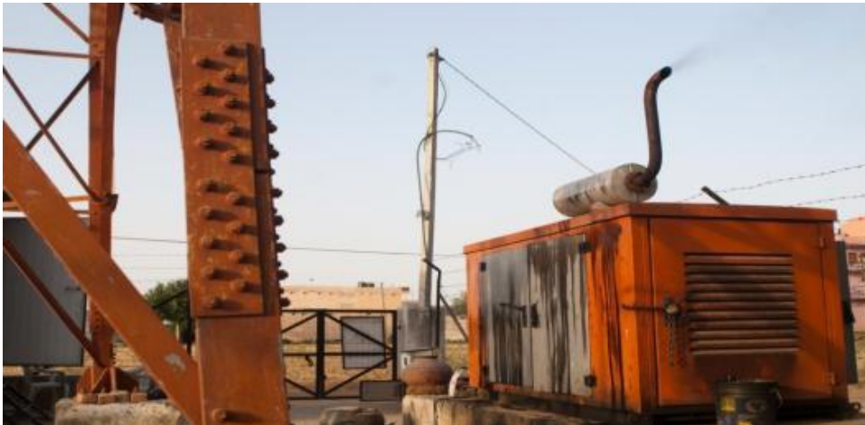
Figure 242: Diesel engine powering a telecoms tower in India 4
