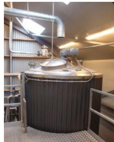
Figure 139: Electrochaea's 250 kW biological methanation reactor for the Foulum project (Danish Biogas Demonstration project) 3
